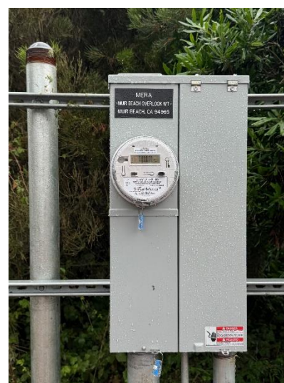
PG&E meter installed at Muir Beach Site.
