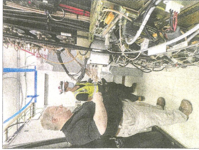
Dave Jeffries (left), deputy executive director of the Marin Emergency Radio Authority, inspects electronic equipment with electrician Phil Chalaris at the Mount Tiburon radio tower on Dec. 1. The radio authority is upgrading its towers with its NextGen system to improve coverage and reliability.
