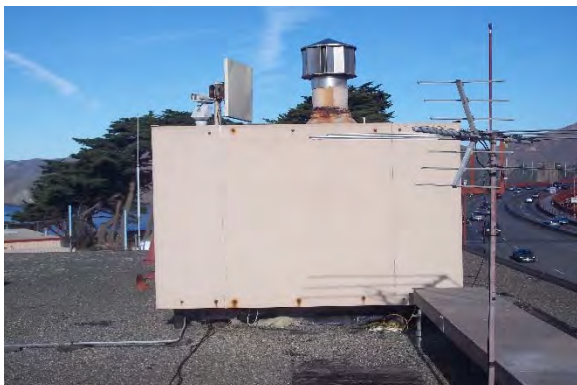
5. Golden Gate Bridge Antenna Pad Exterior
