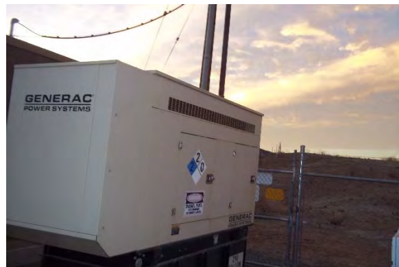
4. Redwood Landfill Diesel Generator
