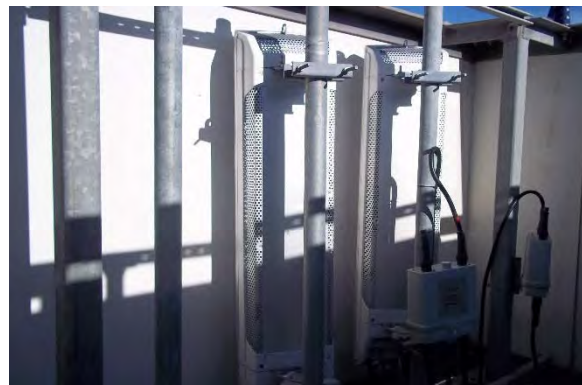
6. Golden Gate Bridge Antenna Pad Interior
